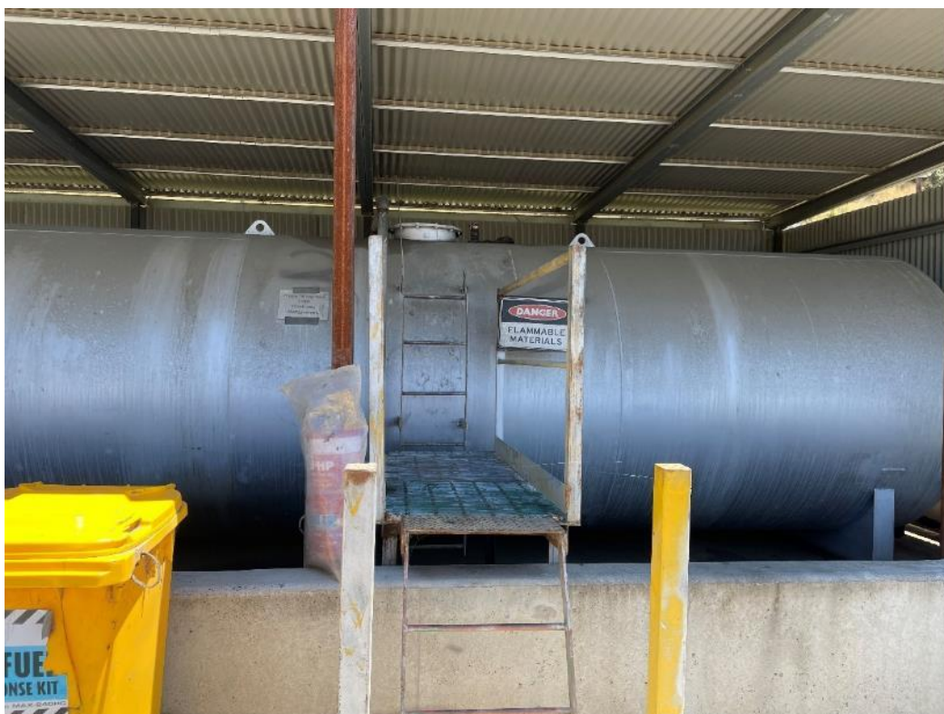
Covered and bunded Bulk Fuel Tank. Spill kit provided nearby.
