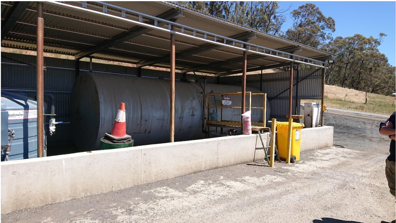
Photo # 4 - Diesel Fuel Storage
